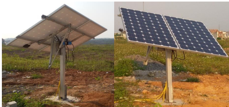
Fig. 7. The real image of the tracking system.
